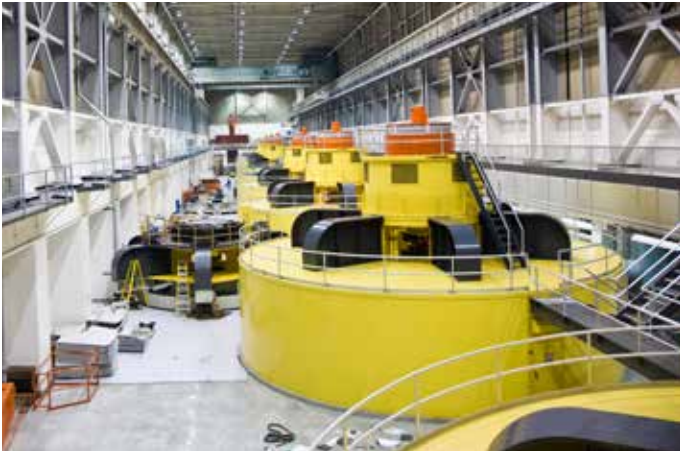
Hydroelectric power generators
