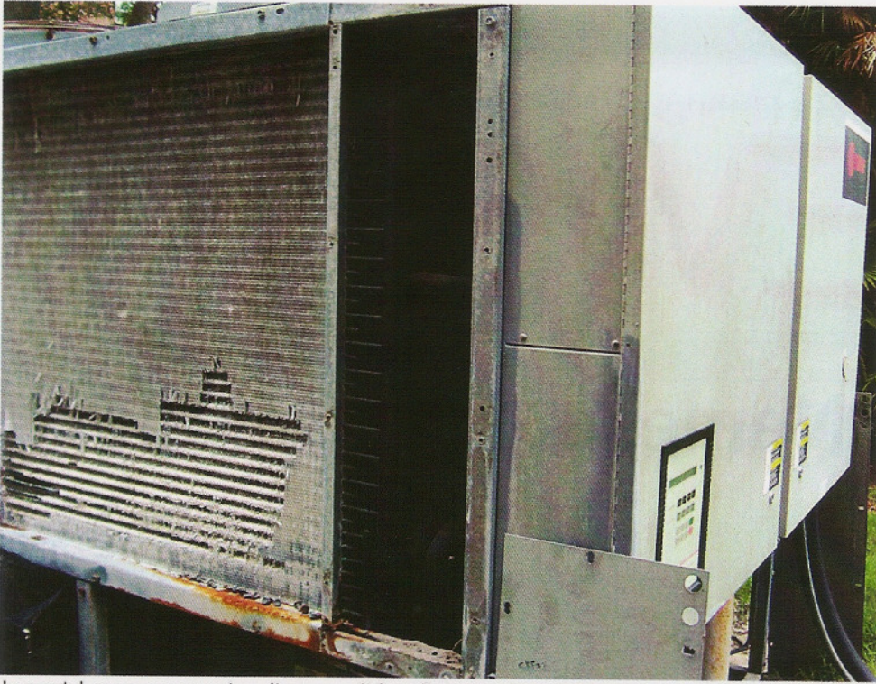
In coastal areas, exposure to salt can result in coil damage that shortens the life of the equipment.
