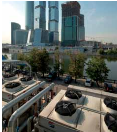
Rooftop-mounted air conditioning units
